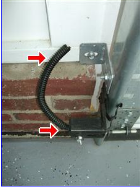
3.3 Picture 1 Control wires in conduit
