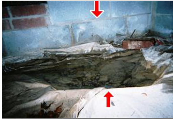
5.0 Picture 1 Up arrow = water down arrow = efflorescence
